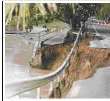
Riverbank slip, Wanganui Source: Wanganui District Council (2000).
